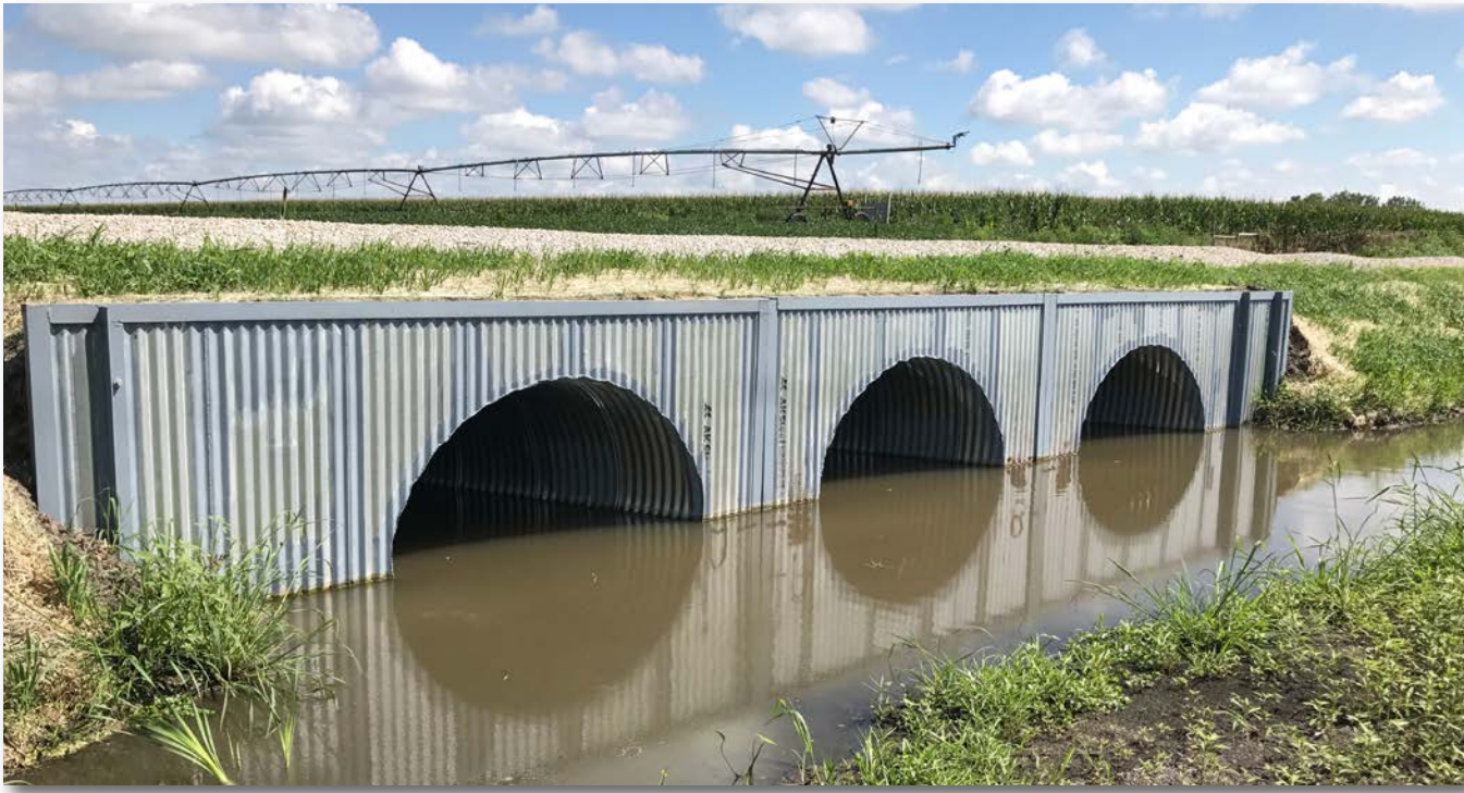
Ohiowa, Nebraska: Triple 71" X 47" Corrugated Steel Pipe Arch on 20 degree skew cut. Headwall reinforced with steel channel and dead man anchors.
