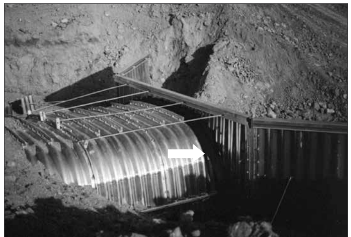
Once the headwall is installed, install fabric behind the headwall where any gapping occurs.
