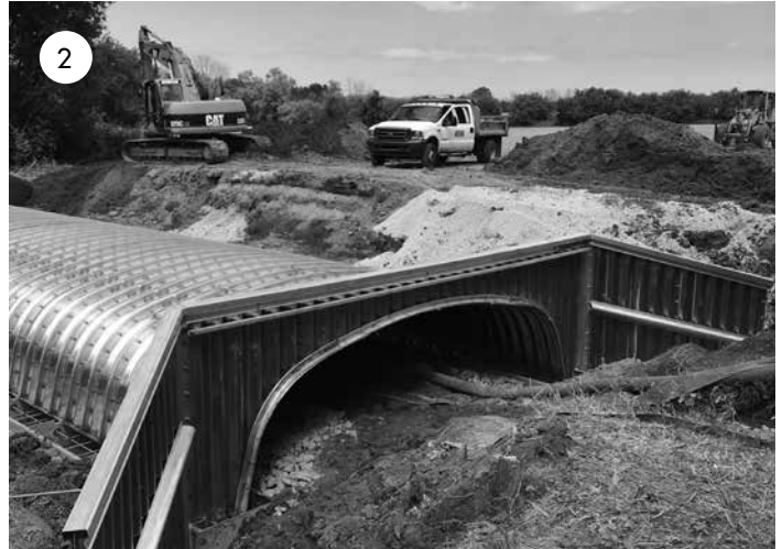
Backfill material is placed carefully before 8" lifts are spread evenly and compacted.
