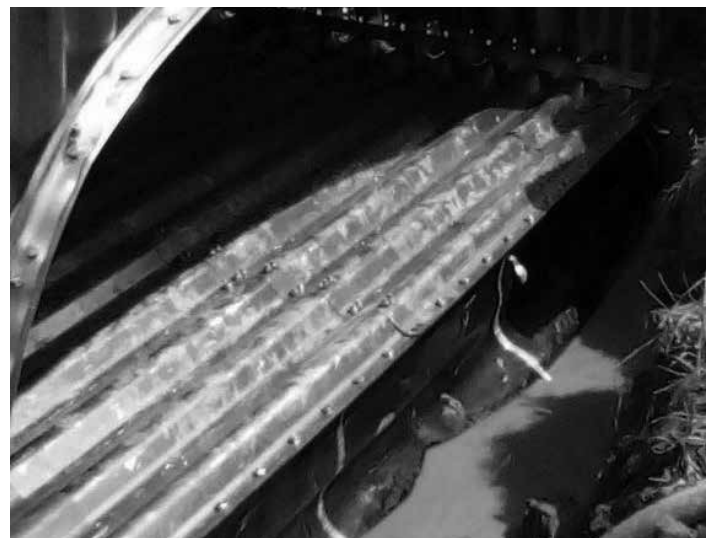
Polymer Toe Wall
